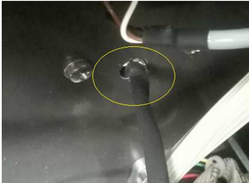
搅拌机电缆的屏蔽线和安装铝板短路
